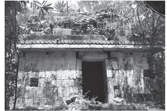
Group 4 structure as it appeared in September 2007, before its subsequent cleaning and restoration.
