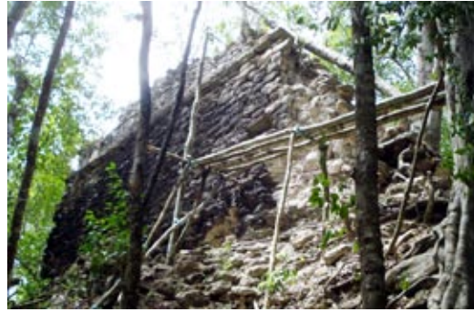
Southern side of Structure A4's temple. All images courtesy of Antonio Benavides C.
