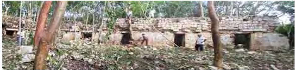
Fig. 3: The cleaning of vegetation and trees on C4-7’s east wing was one of the first activities.
