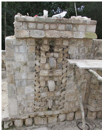
▲ Final result of the restoration of the "Serpents" motifs on the western side of the central room façade of Structure 66.
