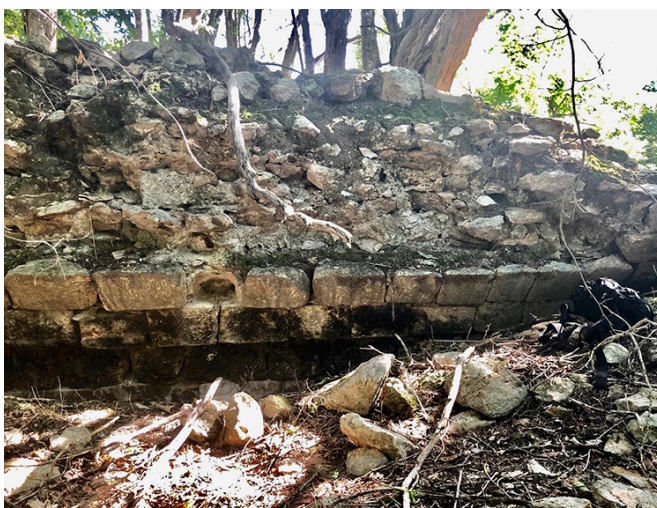
Fig. 2: Fallen front side of one of the central rooms, showing parts of the vault. Photo by Stephan Merk, 2019.
