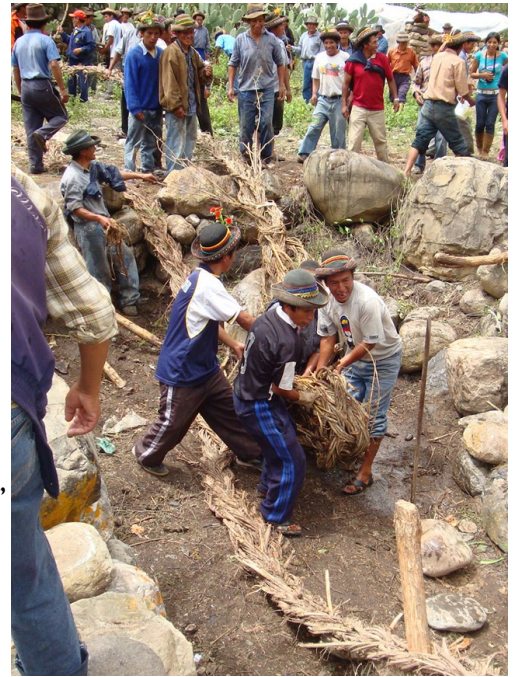
Community members work hard to secure the heavy cables. Photo: Cirilo Vivanco.
